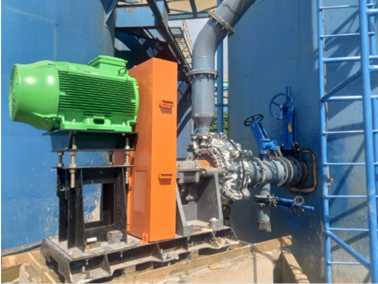
Figure 10: Aachen ® Reactor Installed and Commissioned to Improve Processing Efficiency
