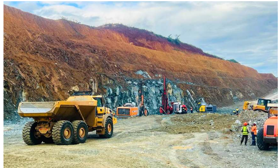
Diesel-powered drilling and haulage equipment operating in the Buckreef Gold open pit
