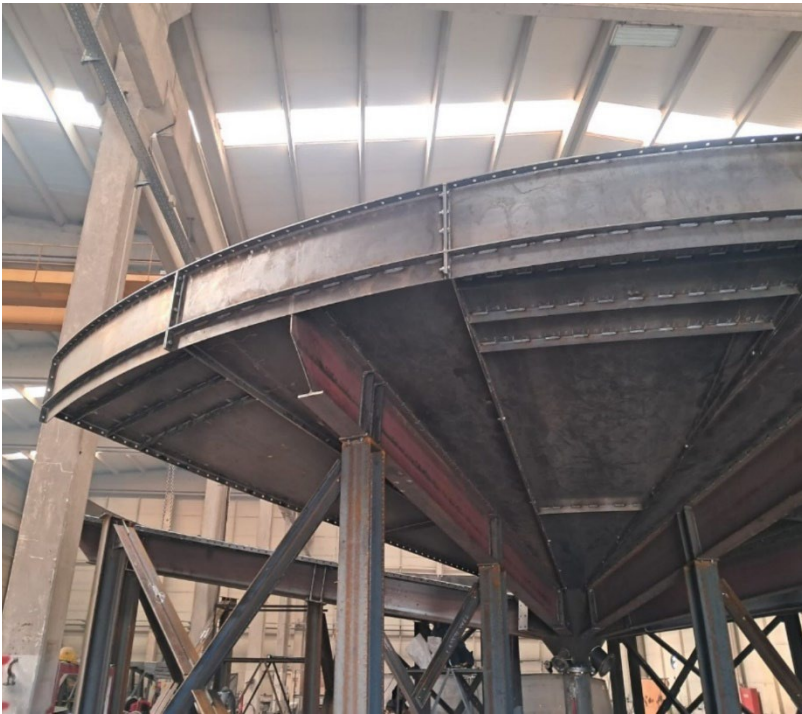
Figures 1a and 1b: 18 meter Diameter Pre-Leach Thickener
